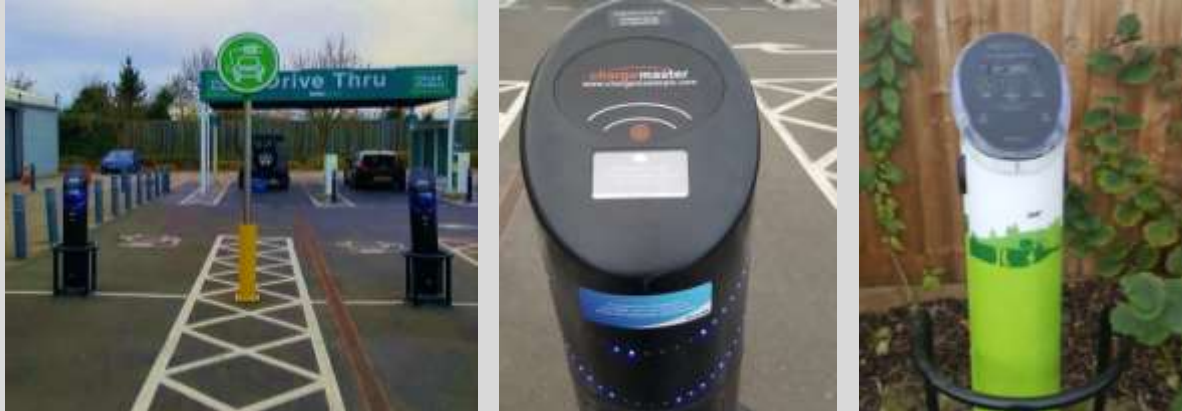
Electric charge points at West Bridgford ASDA and Bingham Lidl's
